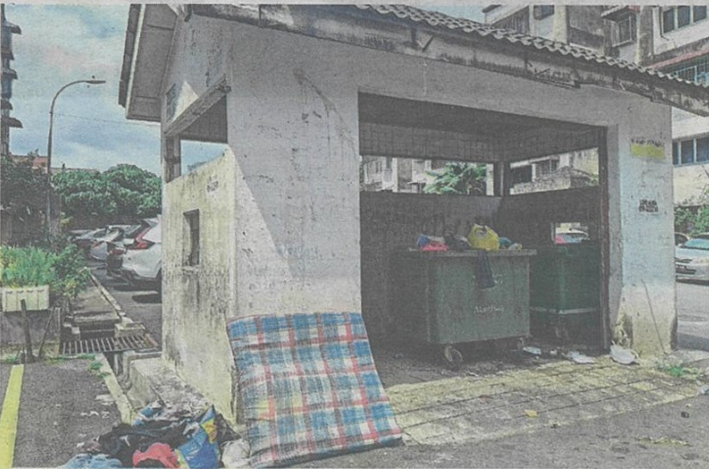
The rubbish chamber at Flat Taman Kobena in Cheras, Kuala Lumpur, has become a frequent dumping ground for outsiders.
